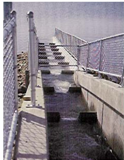
Above: Fish ladder at normal lake elevations.
